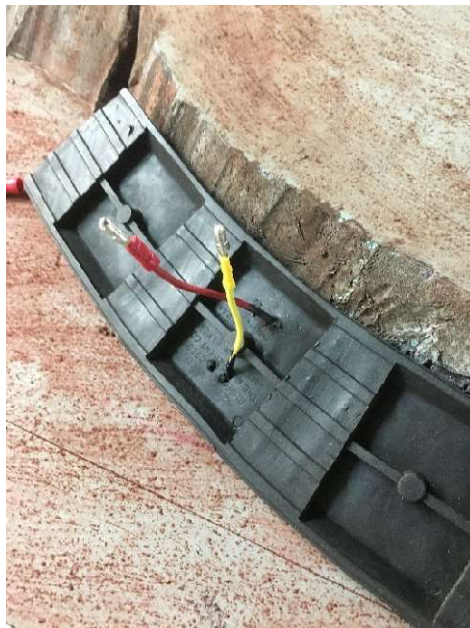
Figure 11 Leads through roadbed with bullet connectors
